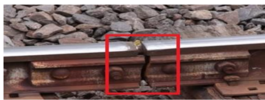
Crack in joint bar
