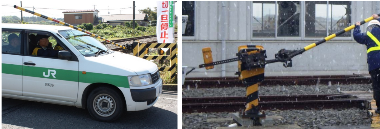
Photo 4: How the crossing gate bends
