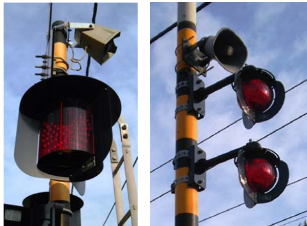
Photo11: Omni-directional type alarm
