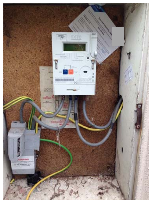
Figure 2: Example of an electricity meter (top) and cut-out fuse (bottom-left)
