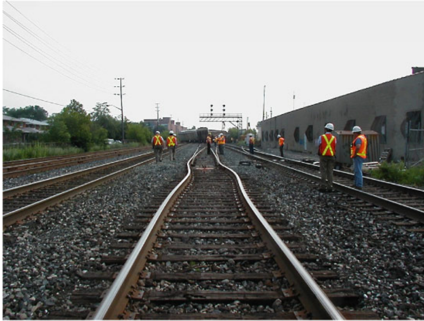
Figure 13: Track buckle in front of the switch of turnout
