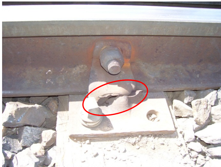
Figure 4: Rail chair broken and creep in the longitudinal direction (Evidence of rail creep within the turnout)
