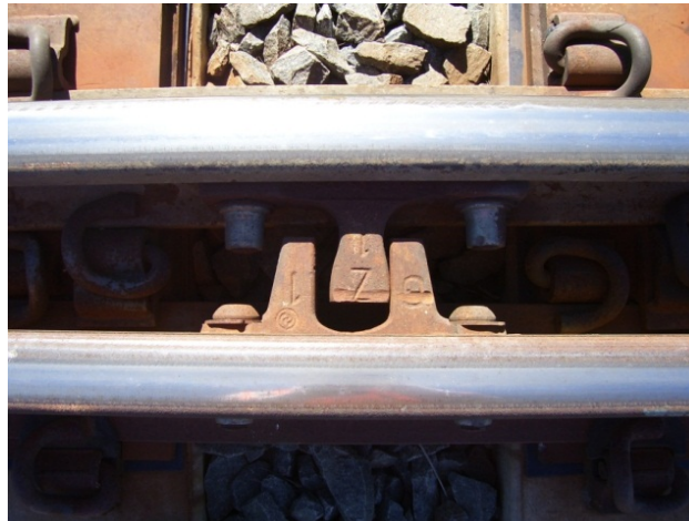
Figure 7: The anti-creep device of Cogifer turnout in the wrong position (e.g. the “T” block very tightly against one side of the “U” block)
