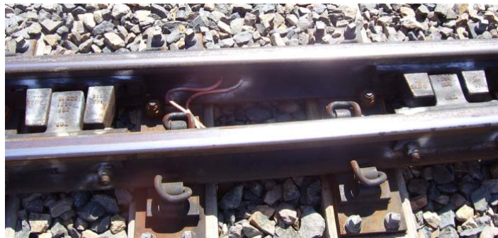
Figure 8: The anti-creep devices of VAE concrete sleeper turnout in the wrong position (e.g. the “T” block very tightly against one side of the “U” block)
