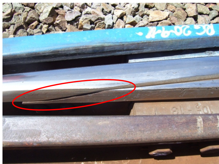
Figure 2: Relative creep (gap) between splice rail and point rail at the crossing area
