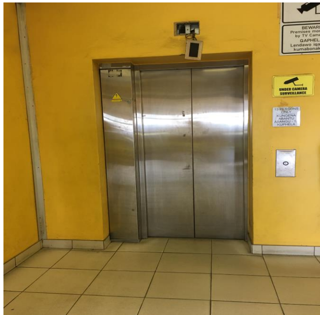
Broken elevator at a station
