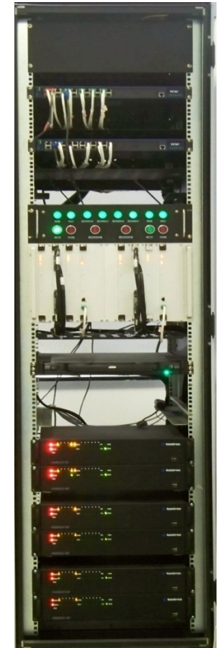
Wayside Equipment of CBTC
