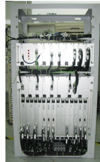
On-Board Equipment of CBTC
