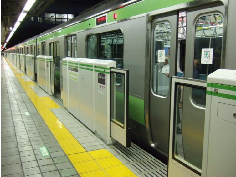
Figure 10: Automatic Platform Gates
