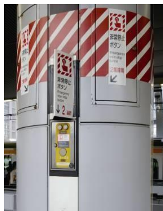
Figure 4: Emergency train stop button
